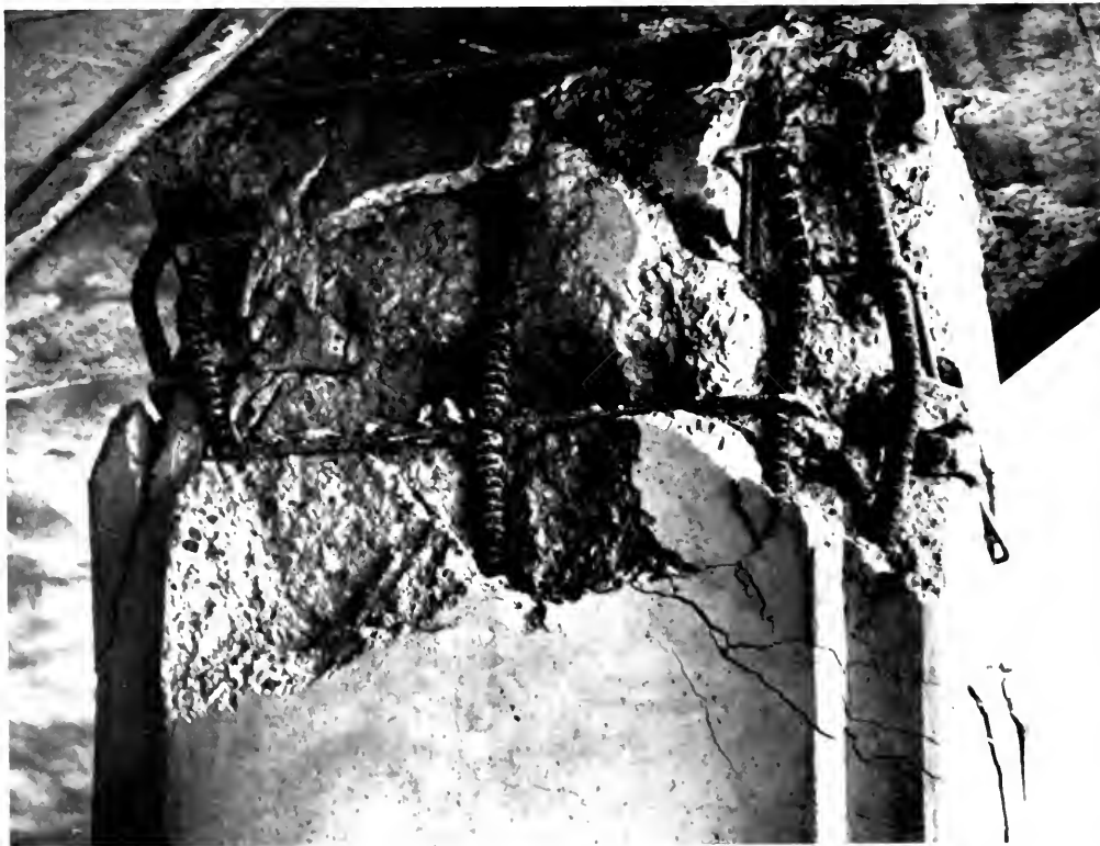
Photo 7. Flexural damage in column of San Fernando Road overhead [2].
